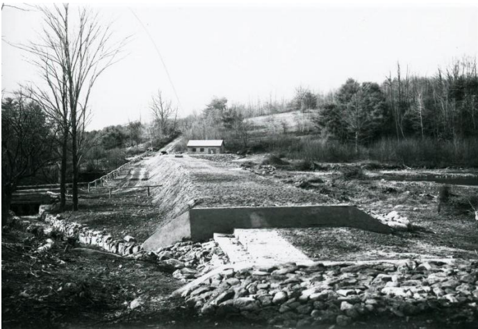
New dam at Woodward Pond, constructed during improvements to the city water system
